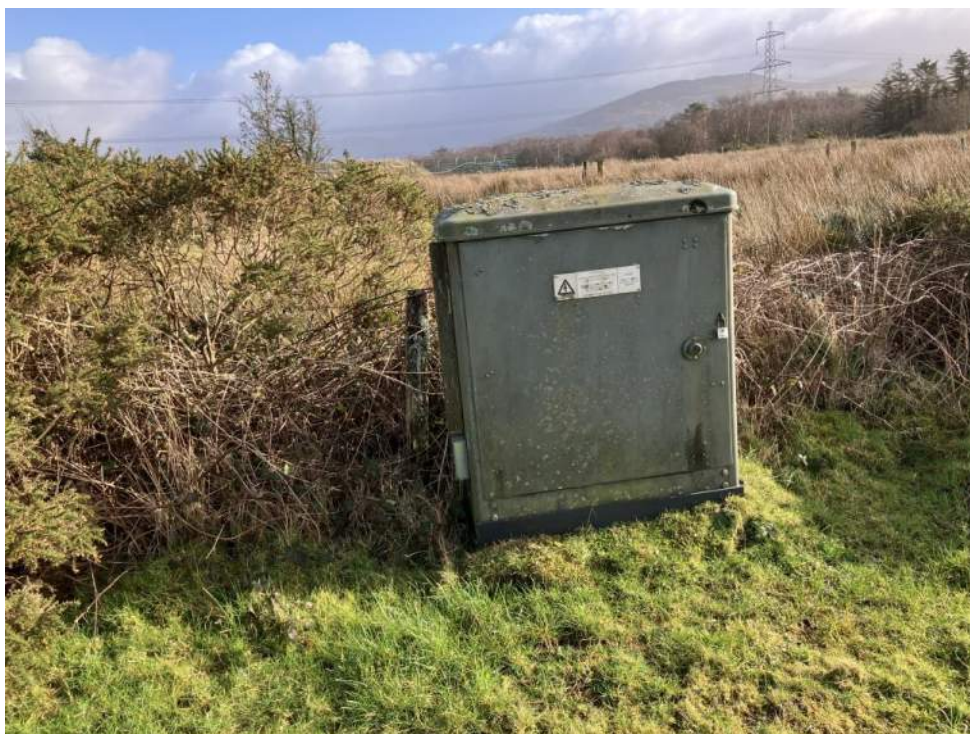
Photograph 15: North-east facing photographs of electrical infrastructure on the site.
