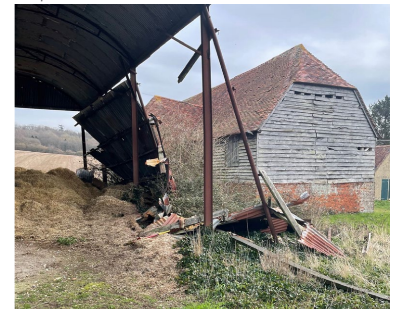
Existing Tithe Barn & Dilapidated Dutch Barn
