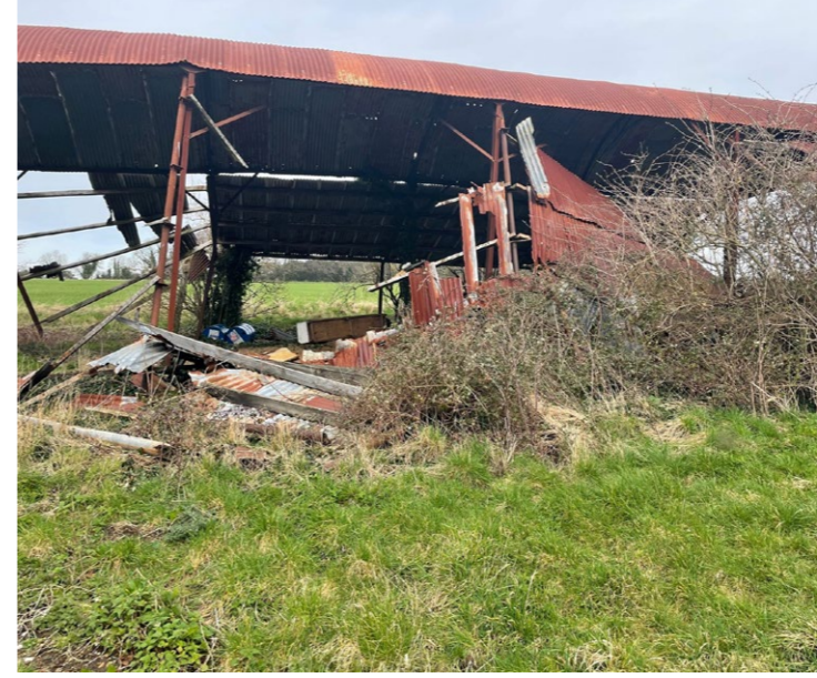
Existing Dilapidated Dutch Barn
