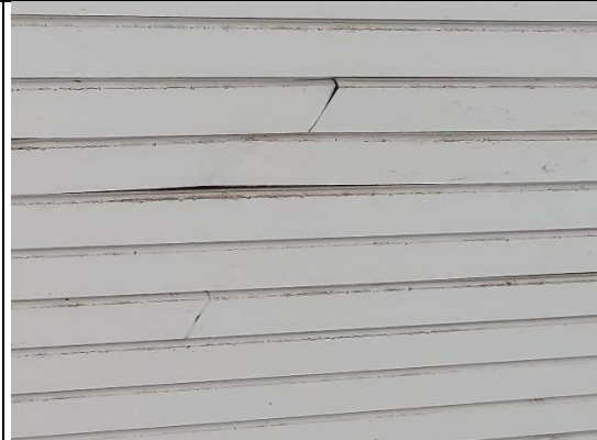
Figure 9 - Warped boarding on building A
