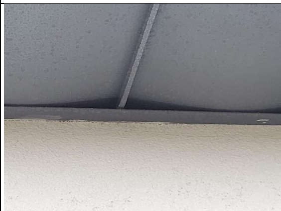
Figure 6 - Warped ventilation covering on building A
