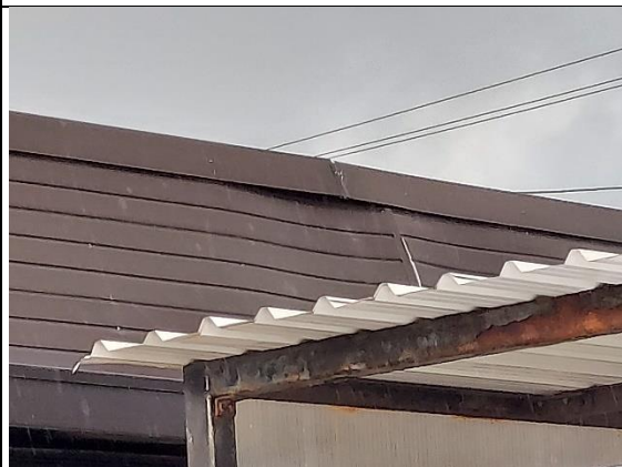
Figure 16 - Gaps in the roof fixtures of building D
