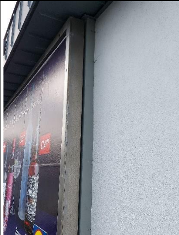
Figure 8 - Gaps behind advertising boards on building A
