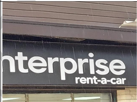
Figure 17 - Hole in the soffits of building D
