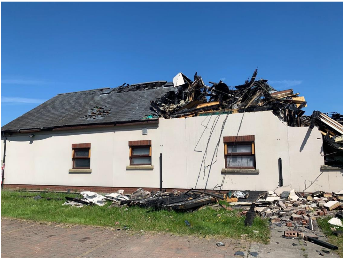
Figure 4: Former Treowen Building – Front Elevation (with fire damage)
